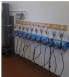
Domeyer filling panels for breathing air compressors
