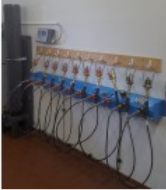
Domeyer filling panels for breathing air compressors Kurzbeschreibung Learn More
